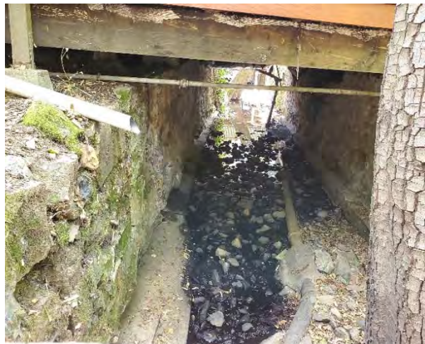
Sections 1 & 2 – Cedar Ravine Creek running under the building and services laterals connected to the 6" CIP sewer main in the creek.
